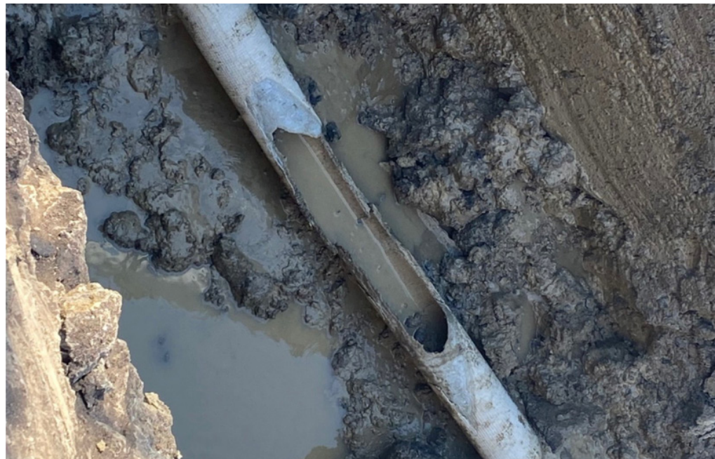
An asbestos cement water main failed in Weyburn, Saskatchewan. The city has approximately 59 kilometres of asbestos cement water mains throughout the city. Photo courtesy of City of Weyburn.
