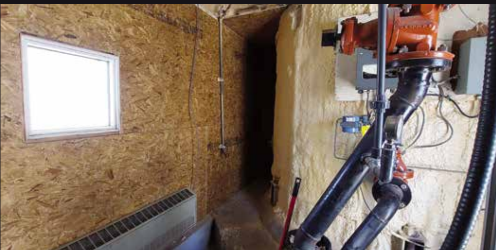
The recent generator installation will help ensure uninterrupted operation of communications equipment and LED lighting during power outages.
