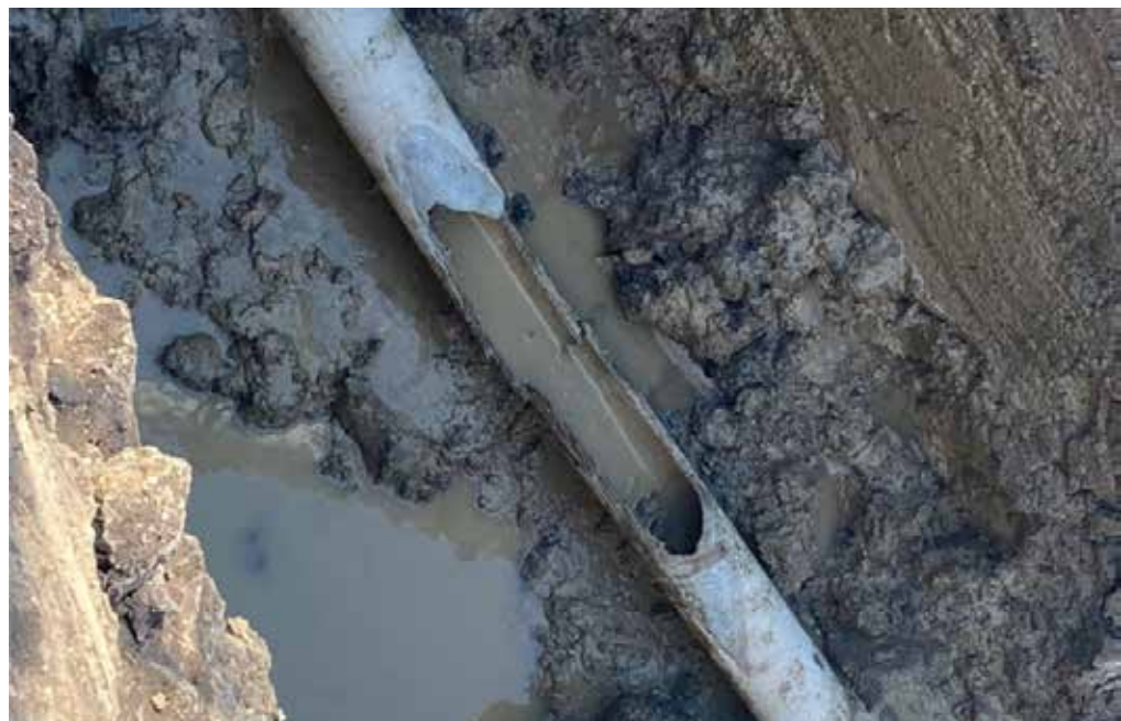
An asbestos cement water main failed in Weyburn, Saskatchewan. The city has approximately 59 kilometres of asbestos cement water mains throughout the city. Photo courtesy of City of Weyburn.
